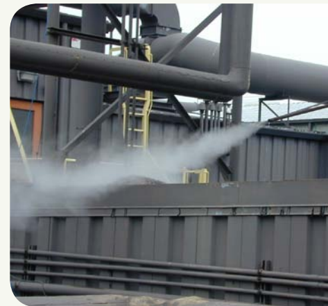
Steam leaks are a loss of condensate and energy
